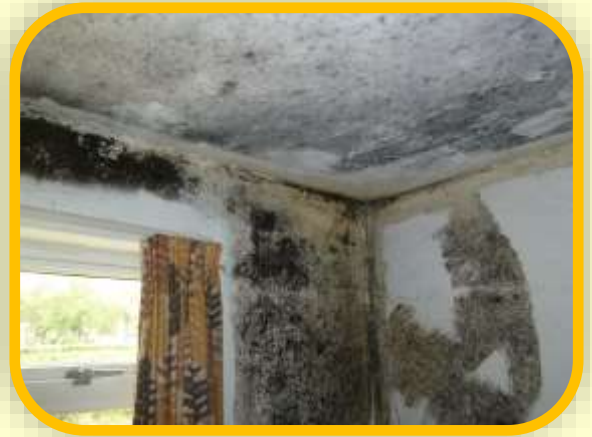
Mould affected home near London
